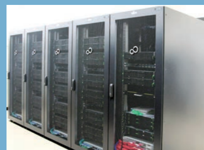
Supercomputer "Flow" Type II Subsystem
